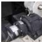
Mechanical overspeed switch
