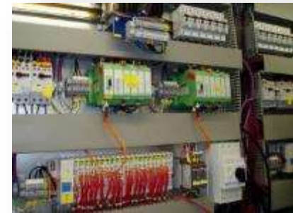
Electronic modules in the switchboard
